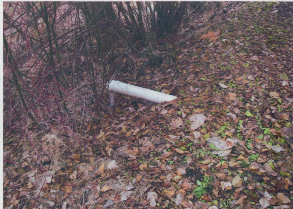
Small outflow below collection box
