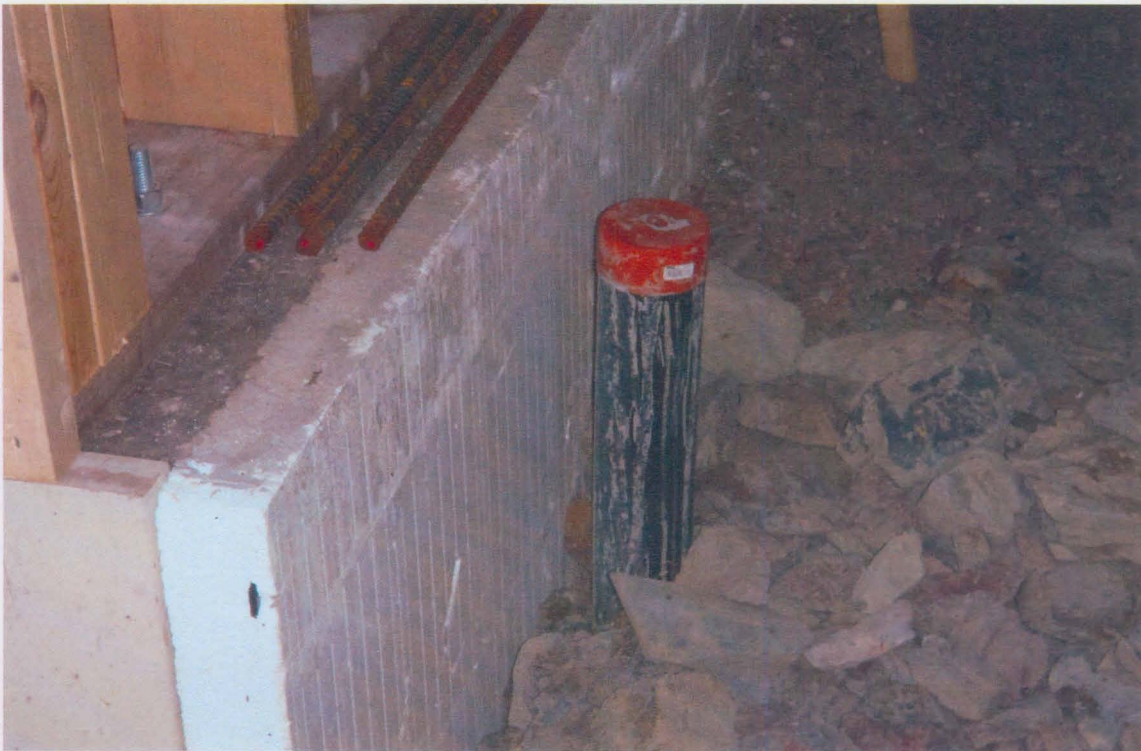
Pipe located inside Jiri+Nada's new dwelling (under construction)
