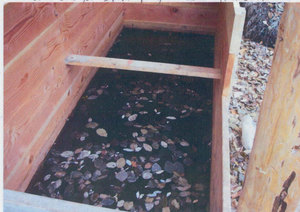
Collection box for Irish Spring. No observed outlet pipe.
