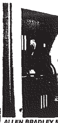
ALLEN BRADLEY MCC'S
