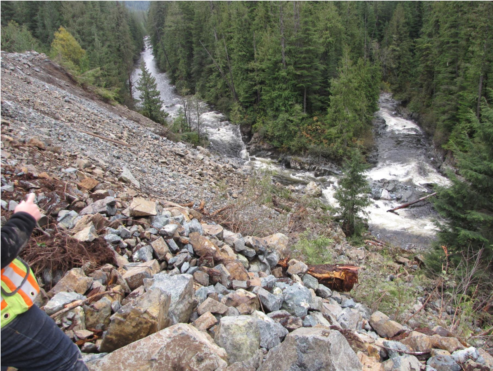
Photo 11 - Blast rock that slid into Kokish River.
