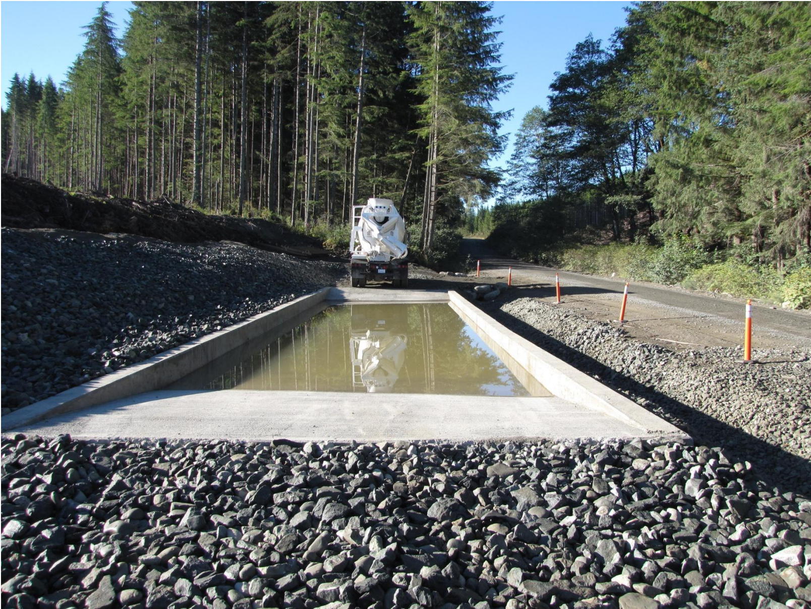
Photo 13 - Wheel washing facility.
