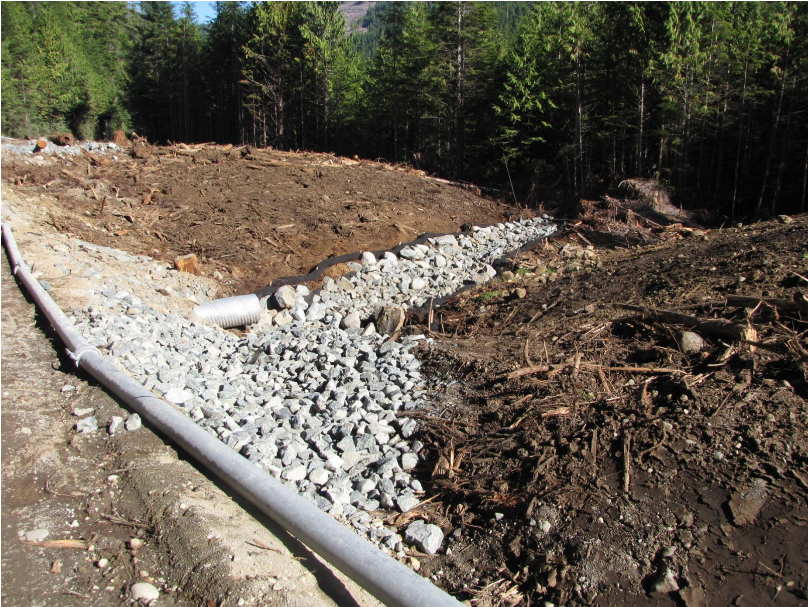
Photo 3 - Rock armouring in stream channel
