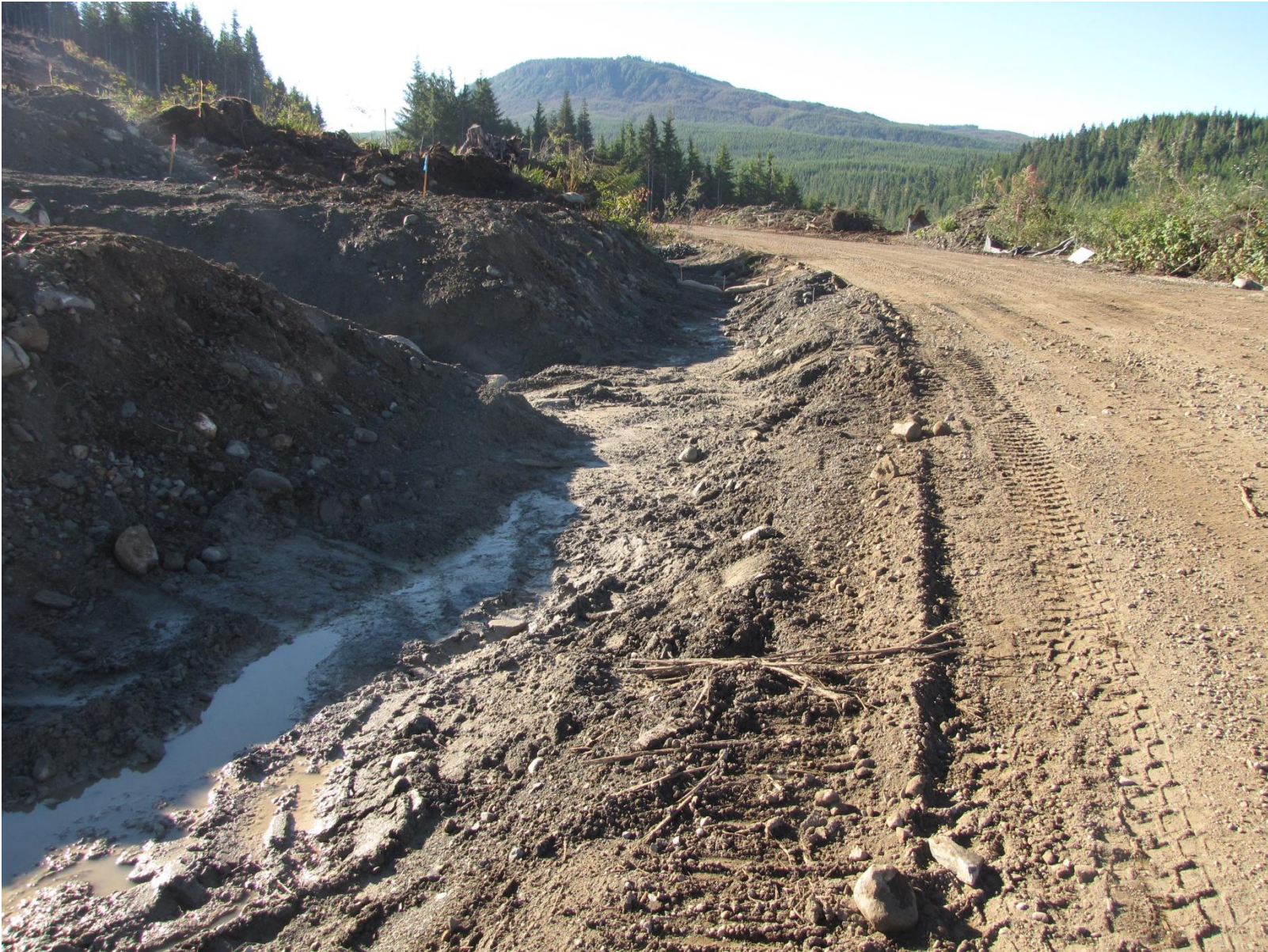
Photo 2 - exposed soil along Kokish Main road
