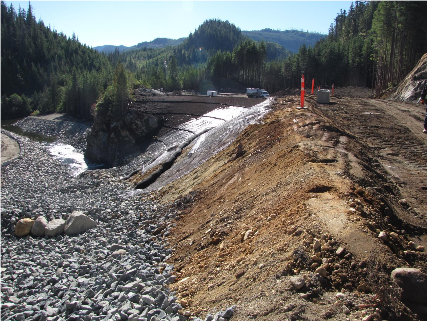
Photo 4 - Hydroseeding over geotextile mesh with compost mixture for slope stability and erosion control
