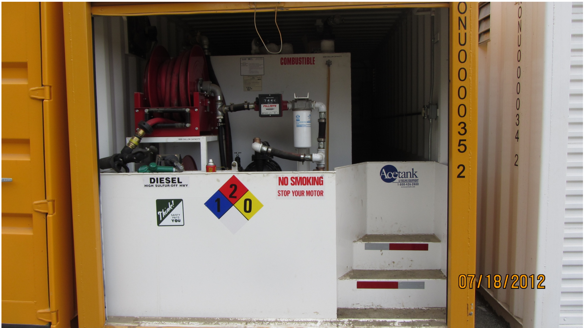
Attachment 6 - Fuel storage tank labelled as "high sulphur - off hwy"
