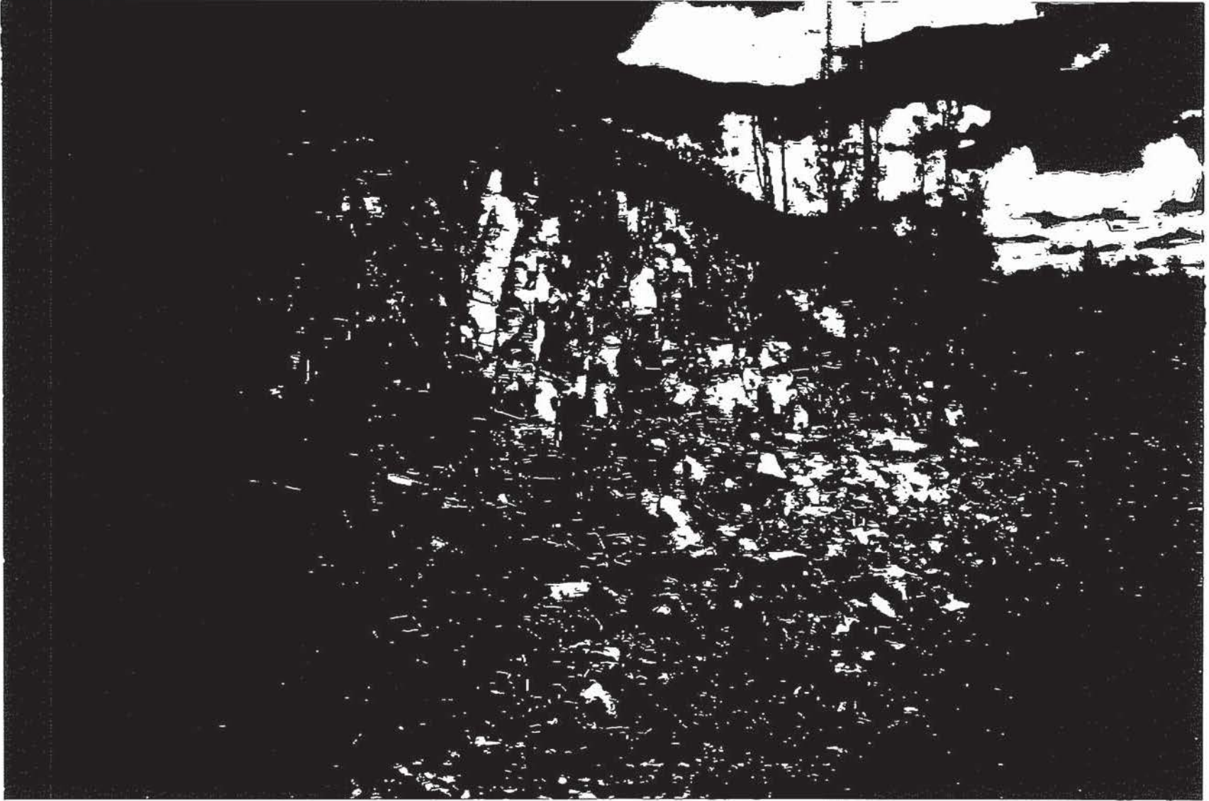
Photograph 3: Raveling typically occurs on Southwest Wall.
