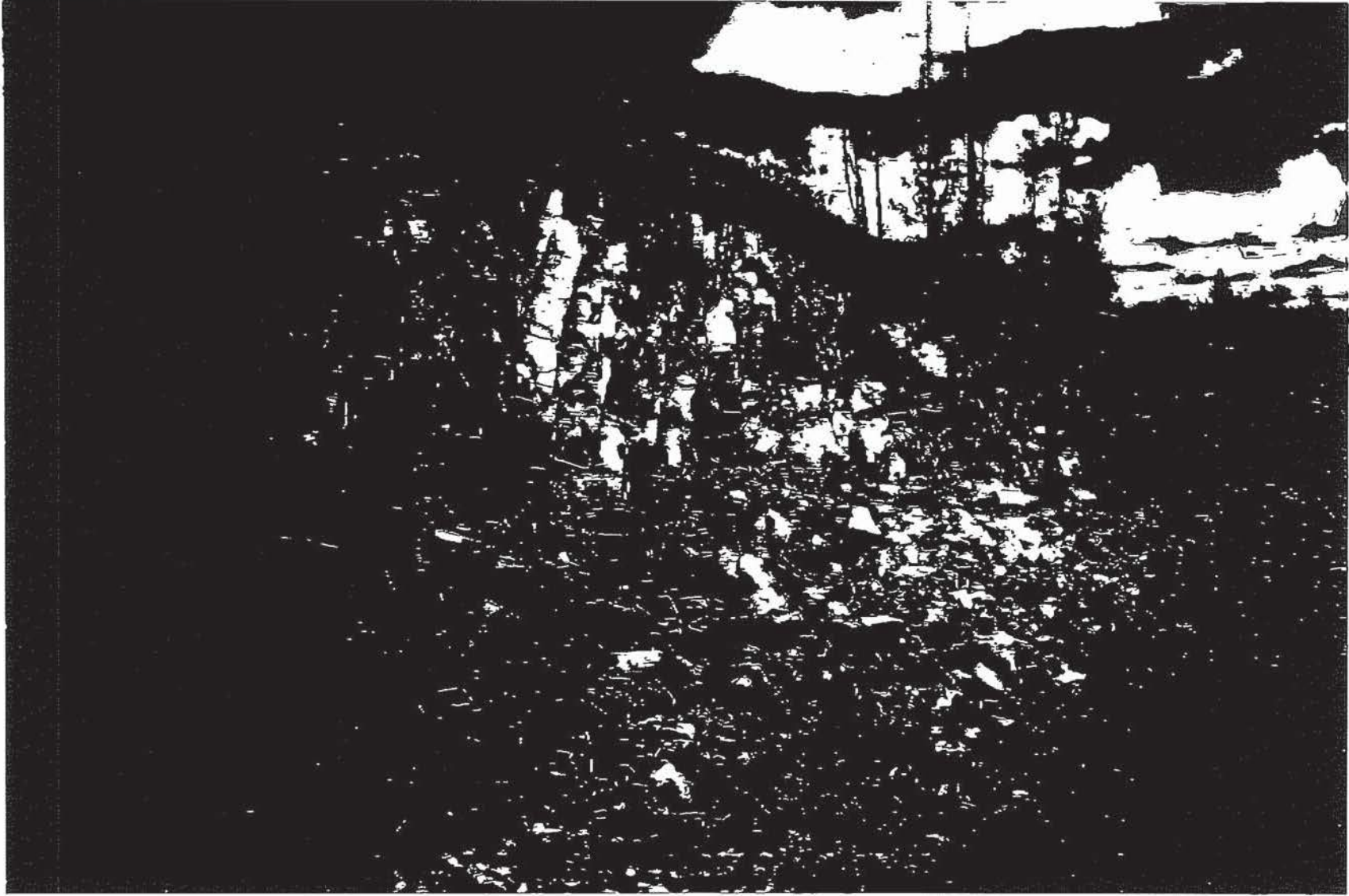
Photograph 3: Raveling typically occurs on Southwest Wall.
