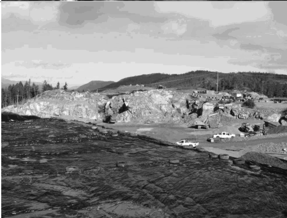
Looking north across Encapsulation Cell 1A at the north side of the quarry. The unstable area discussed in Field Rvw Rpt 1 is behind the red rock crusher.
