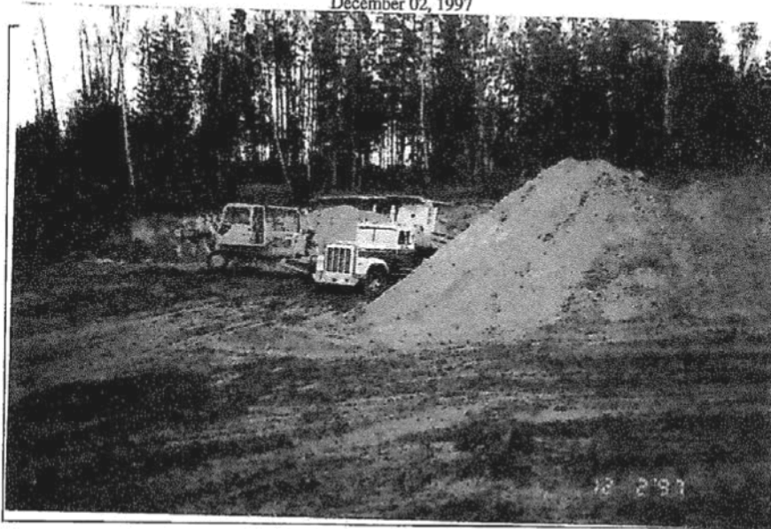
PR 11191 BZ Enterprises Ltd Landfill site, Salmon Arm, BC December 02, 1997
