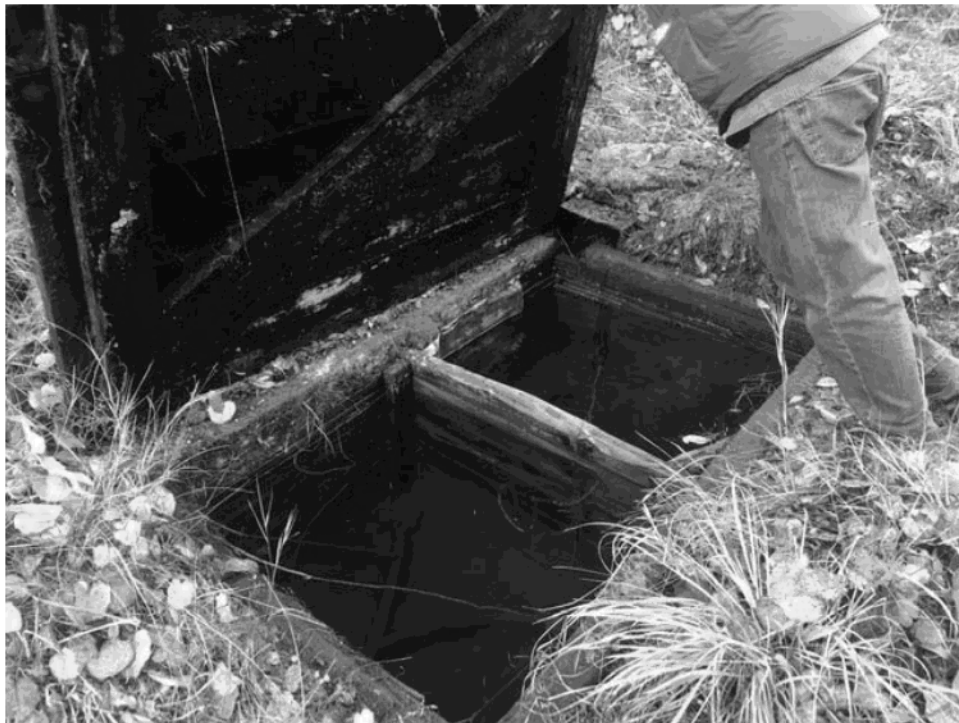
Photograph 6 – Interior of Davidson Spring water box. Sample WB-1.
