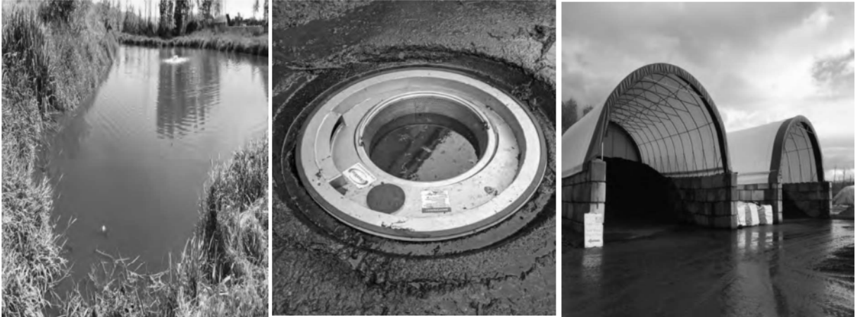
Existing Storm Water Pond w Surface Aerator / SW catch basin screen / Compost Storage Tents
