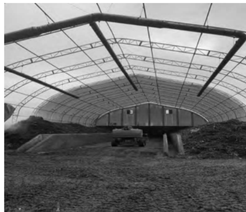
Building Roof Holes and Separation 7 years old / New Roof Installed October November 2019
