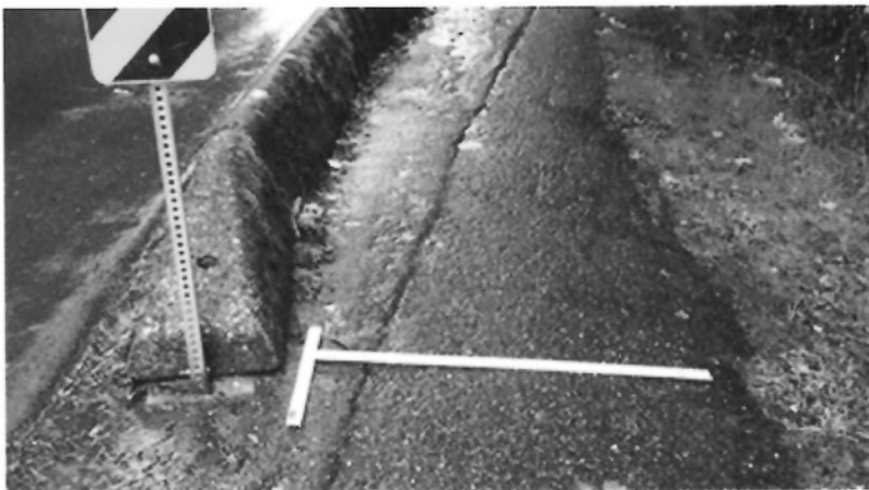
Figure 3: 'Sidewalk' width at access point less than one meter
